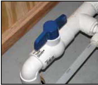
Drain valve for fresh water system. Shown in "open" position.
